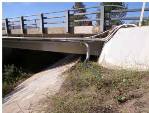
Utilities located on the bridge will require staged relocation to maintain service during construction.
